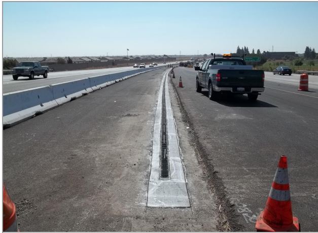
I-5 Median Slotted Drain - Elk Grove area
